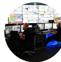
Security Operation Center
